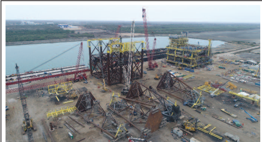
Engineering, procuring, constructing and installing large offshore facilities is a complex and multifaceted process. Digitizing and standardizing engineering and construction activities drive down project costs by eliminating legacy systems and simplifying processes within a single integrated platform that can be leveraged from the point of inception of a project's design to its eventual decommissioning. This photo from a drone gives a view of the 2,300 metric-ton jacket and four tripods, as well as the 14,500 metric-ton topsides, for the Pemex Abkatun A2 Bay of Campeche project during fabrication.
