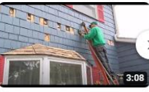
Blowing Cellulose Insulation in a Home with Shake Siding 48 views · 6 months ago
