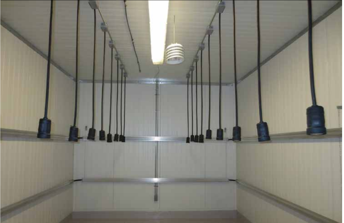
Acclimation chambers with electrical supply for rolling racks, two rows of StarFin™ along perimeter walls.
