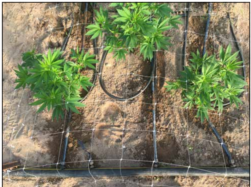
MegaTube loops and supply pipes exposed near the surface of a raised bed.
