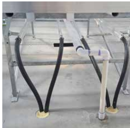
Balanced CO2 distribution with BioTherm's DuoFin™ under-bench system.
