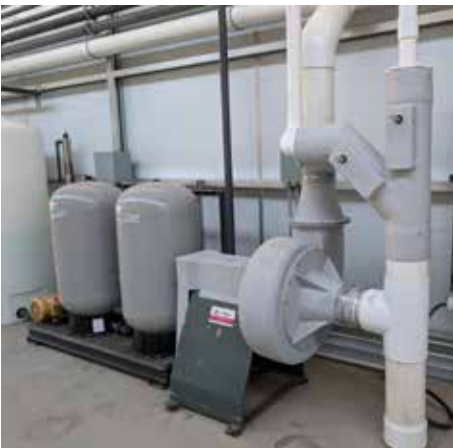
BioTherm's highly efficient Co2 Enrichment system in use.
