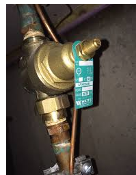
Watts regulator leaking... reddit.com
