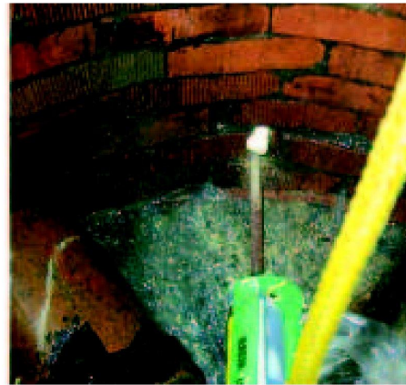
Aqua Seal Stopping Leak
