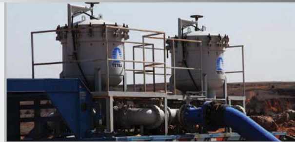
Filtration to Remove Particulates
