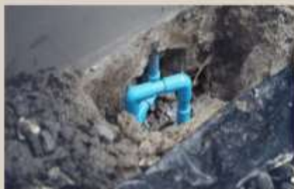
BROKEN PIPE UNDER SLAB
