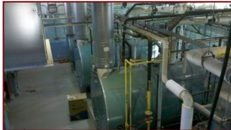
V.A. Medical Center - Combined Heat & Power
