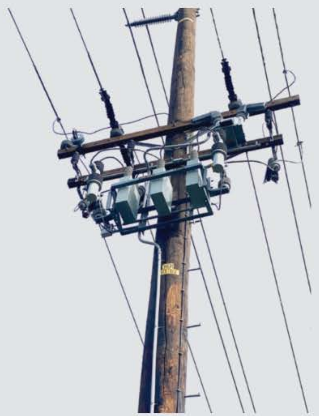
Pole-Mount Capacitor Banks
