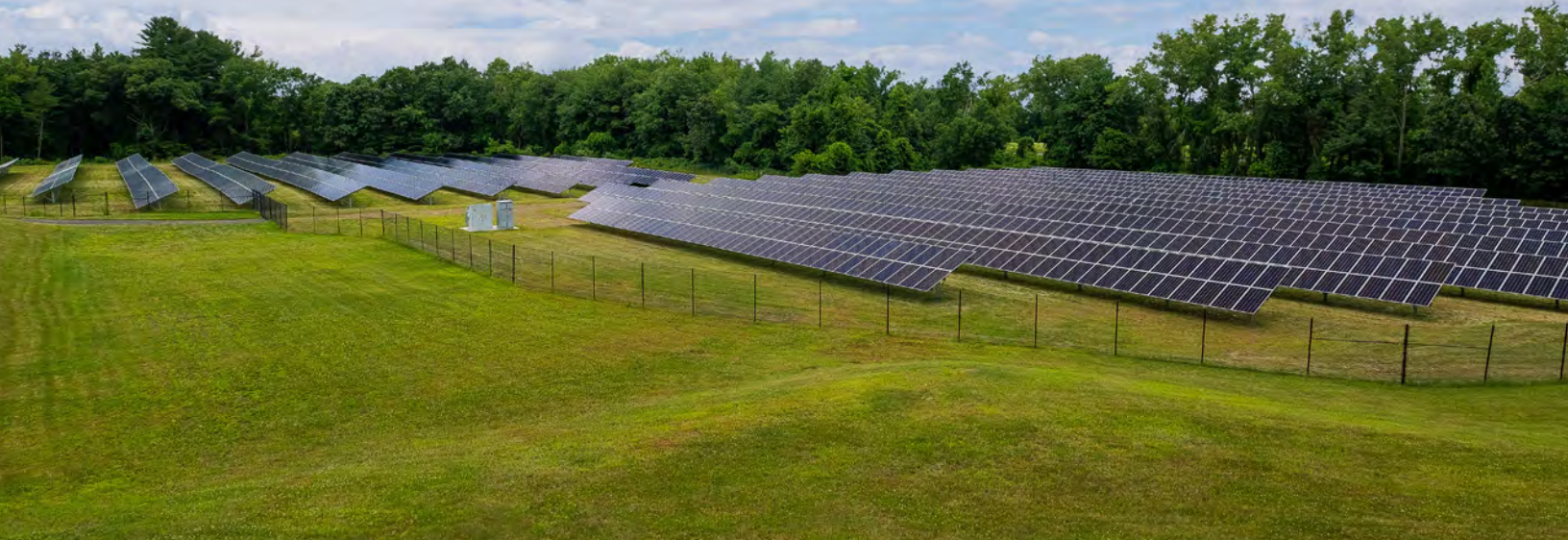
DSD's 2.7 megawatt ground mounted solar project for Manchester Community College in Manchester, Connecticut.
