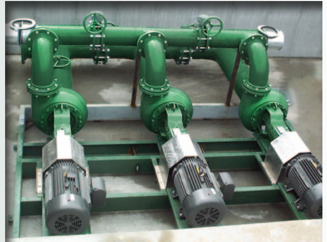
GreenLine 10X8X14 Flush pumps for 24,000 cow dairy with back-up pump.
