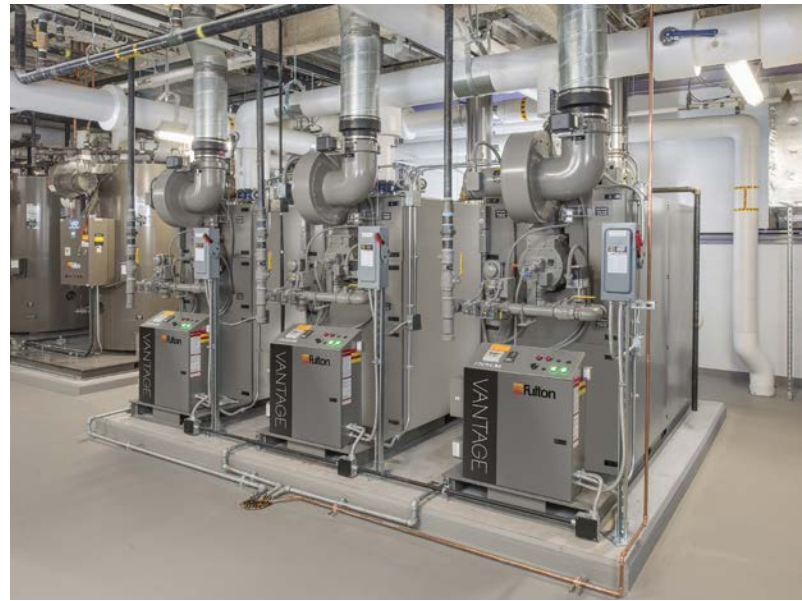
▲ A healthcare facility in Wisconsin utilizes three Vantage 3.0 MM BTU/hr boilers for multiple heating applications
